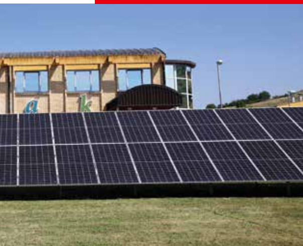
Jazak drinking water production plant
