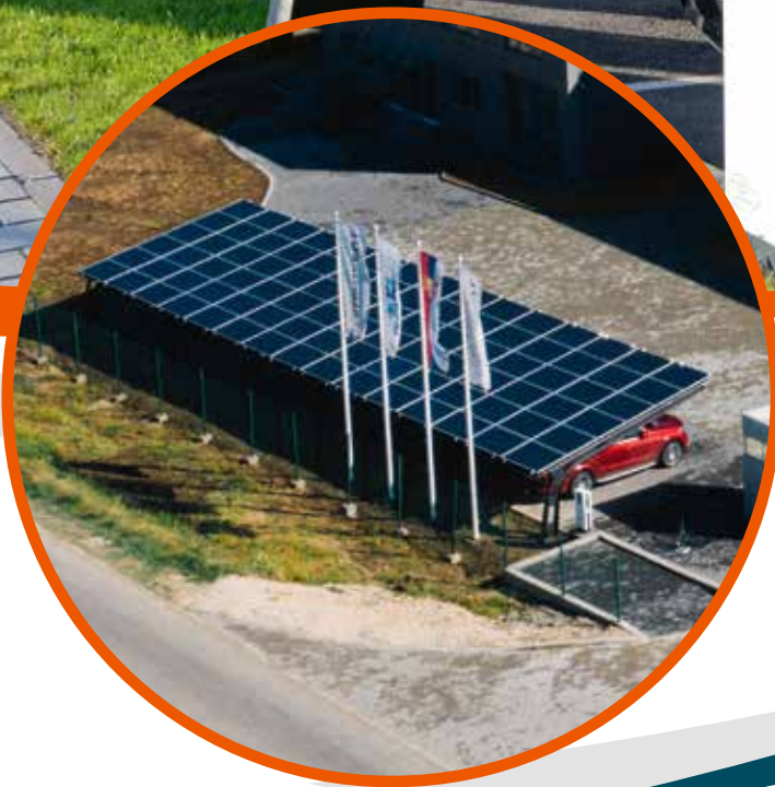
Carport with 10 parking lots and solar power plant with 24,75 kW capacity
